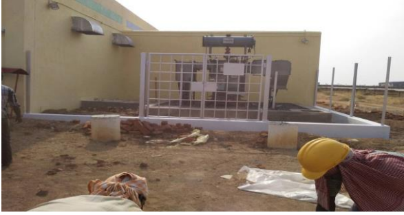
FENCING OF TRANSFORMER NARIKUDI
