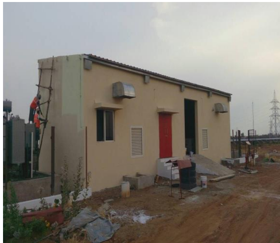
INVERTER ROOM FOR GREENKO TOTAL 16 NOS
